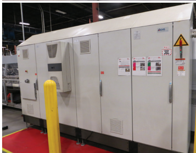
The above images show safeguarded equipment in PepsiCo Beverages Canada’s Mississauga Falbourn Plant. PHOTOS COURTESY OF PEPSICO CANADA.
